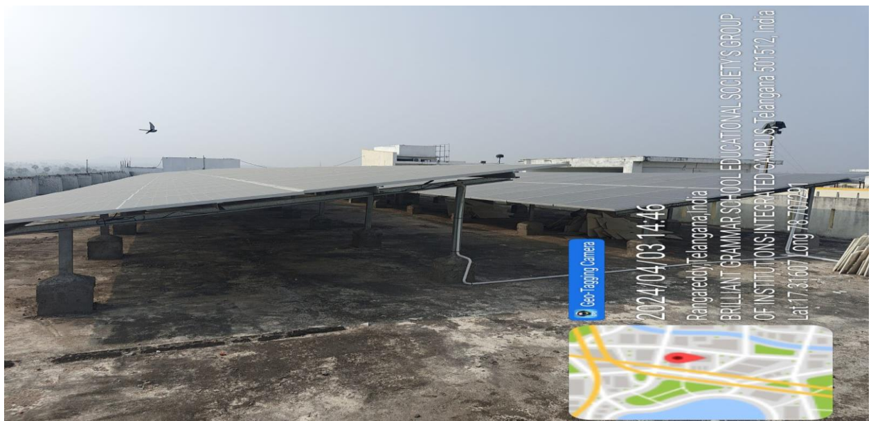
View of Solar Power plant 75 KWp.
