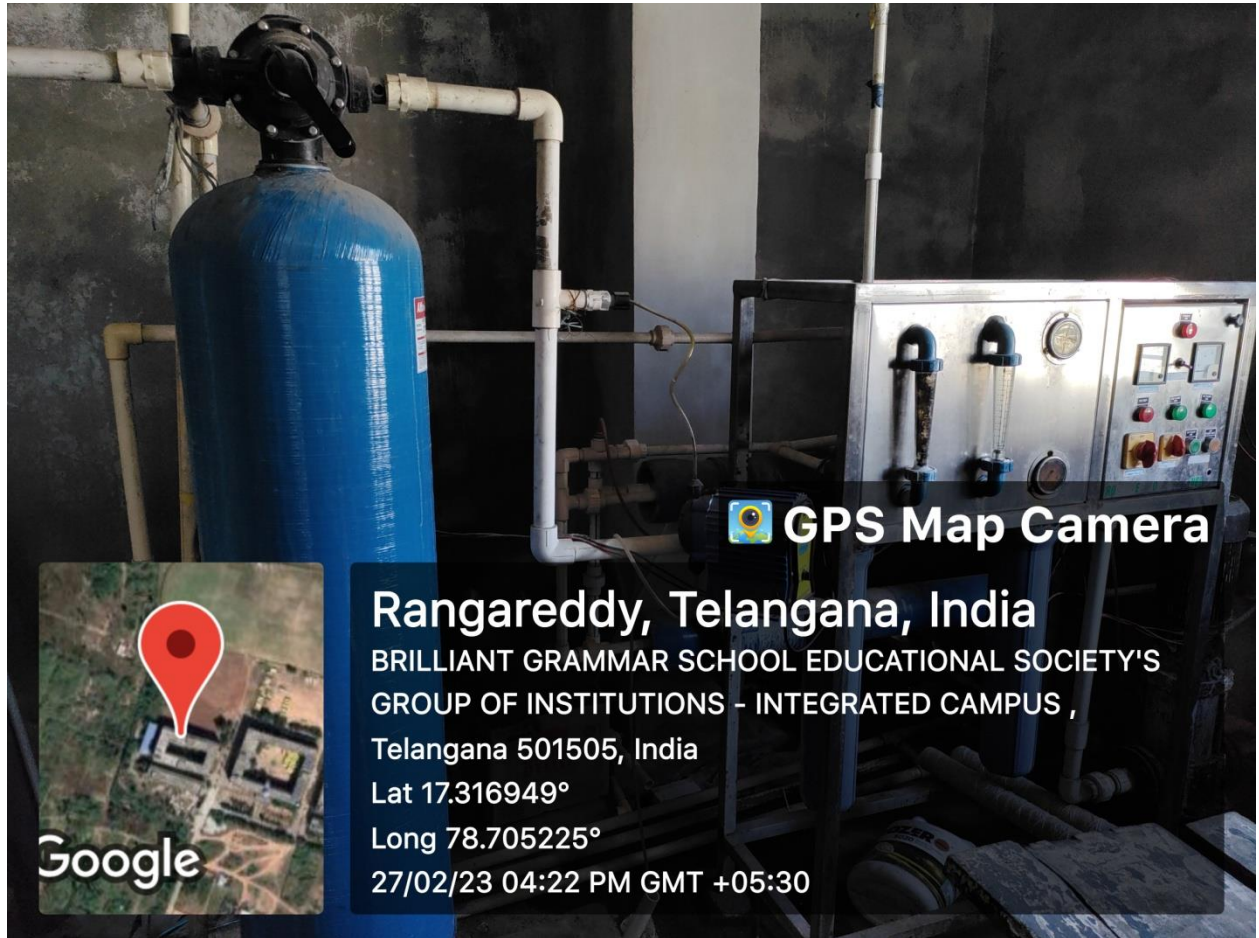
RO water plant.
